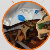
ELECTRIC GROUNDING CONNECTIONS, PLUMBING & GALLEYS
