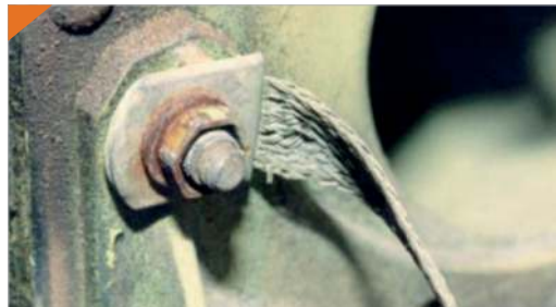
FIG 3: CORRODED BONDING STRAP AND CONNECTION (FROM FAA AC 43-206)
